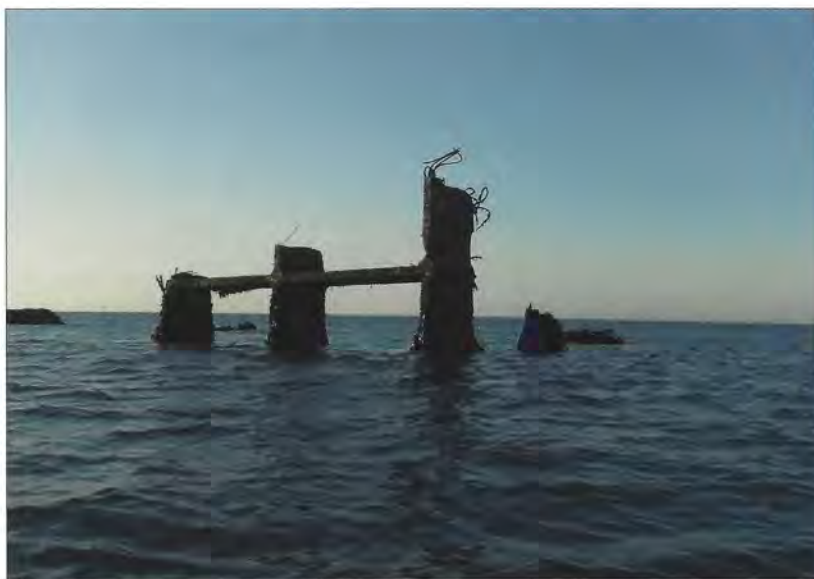
Some of the dangers that remained submerged at high tide but became exposed at low water. The vertical concrete structures and extruding rebar constituted a very real danger for the survey boat.
