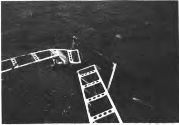
Figure 15: This tower failed due to "human factors!"
